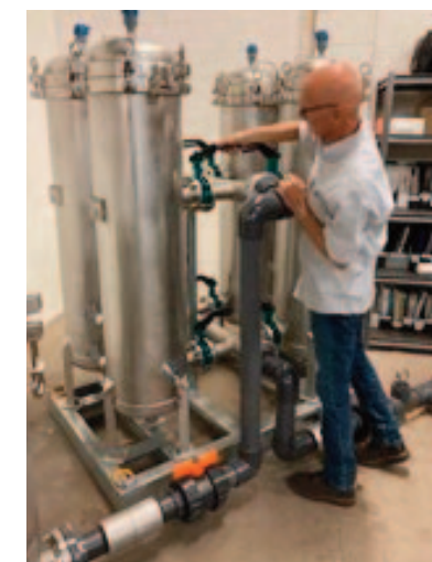
50 GPM Skid with single-bag prefilter and piping sub-assembly.
